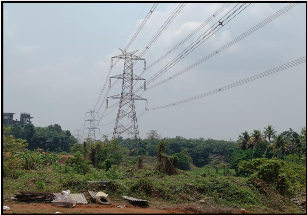
Present status of the KSEB high tension line in the project site
